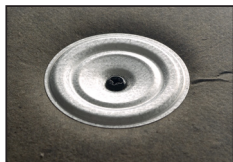
Incorrectly installed, overdriven plate/fastener.
